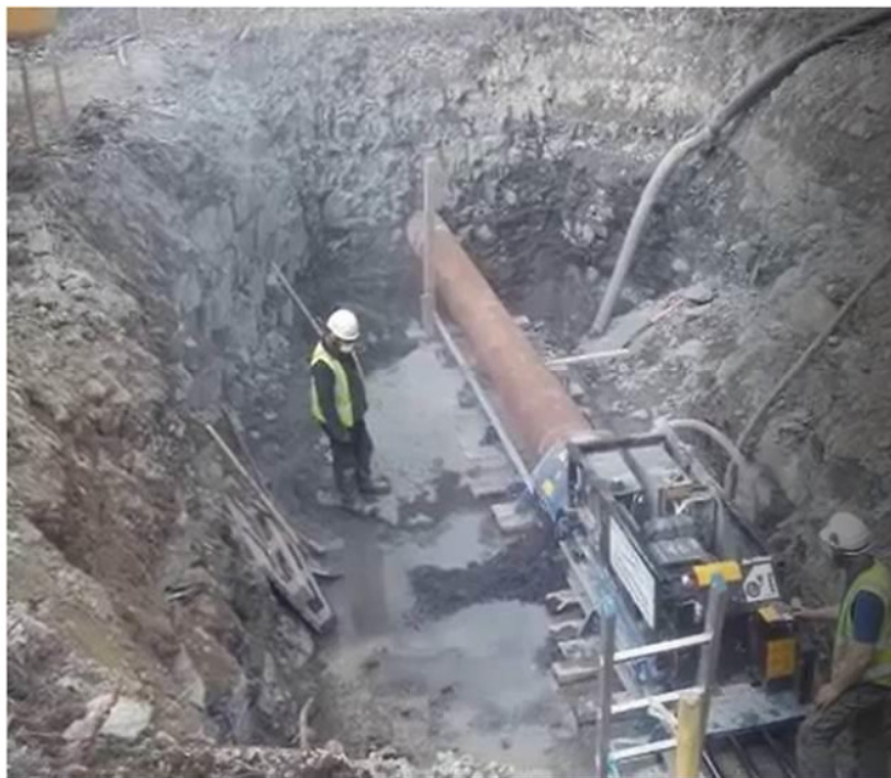
Figure 13 – Auger boring rig setting up to drill a 508mm steel casing with a DTH hammer.
